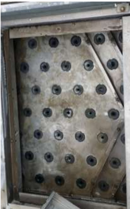
Scale blocked cooling water passage at tower top
