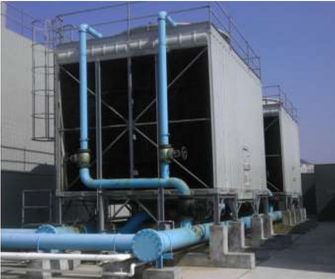
Cooling Water Tower
