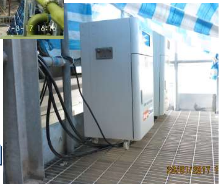
Controller Panels and cable entry
